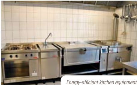
Energy-efficient kitchen equipment
